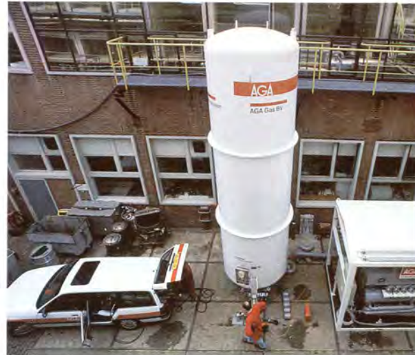
Experimental refrigeration system in Oss, the Netherlands, is to limit pollutant emissions into the atmosphere.
