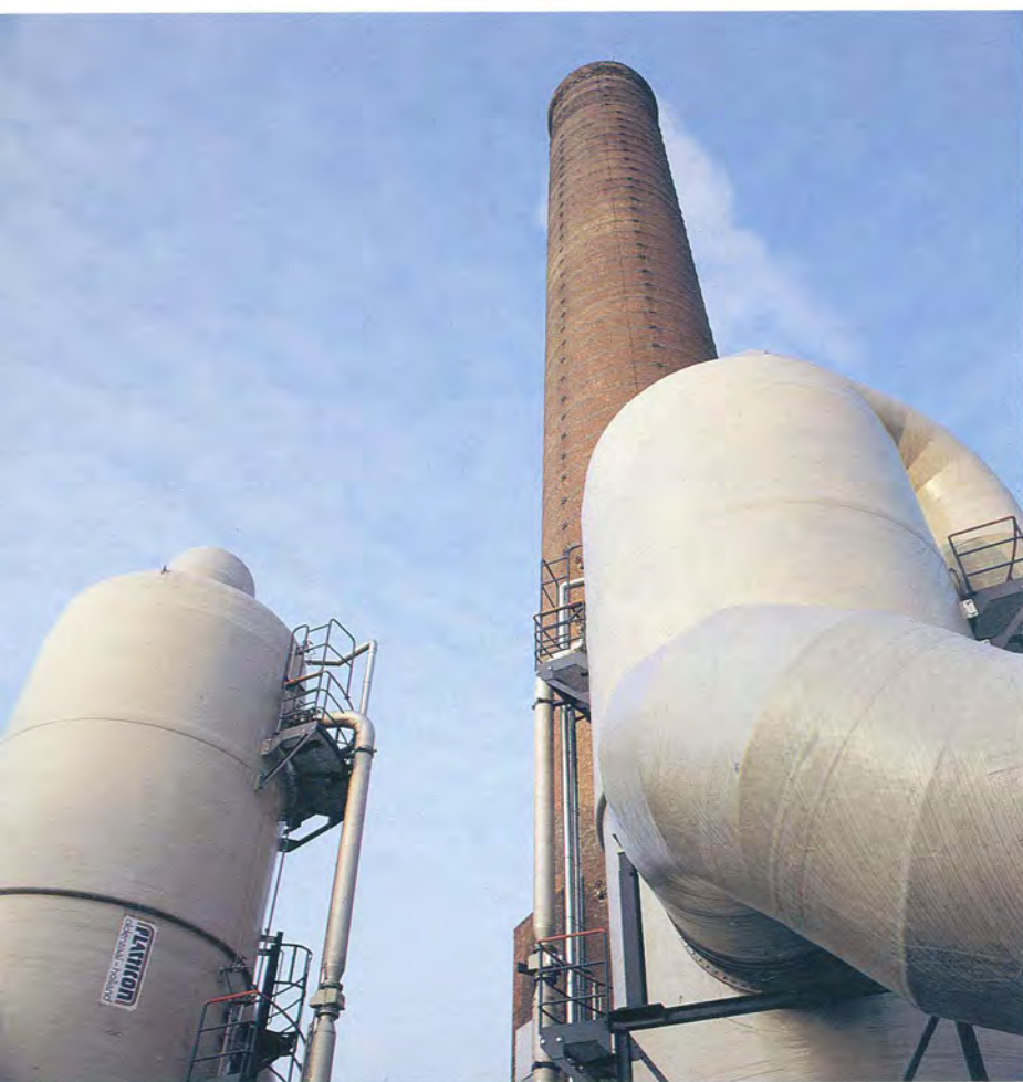
Scrubber installed at the Ede, the Netherlands, site reduces emissions of pollutants.
