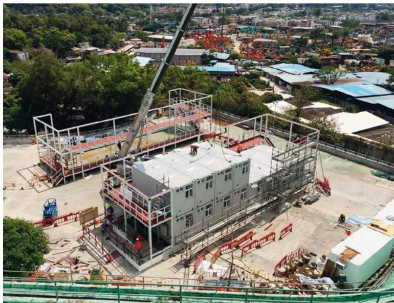
Although Mainland China was still in partial lockdown at the time, we reacted swiftly to supply essential products and services, enabling the Pak Heung emergency quarantine facility in Hong Kong to be completed as quickly as possible.
