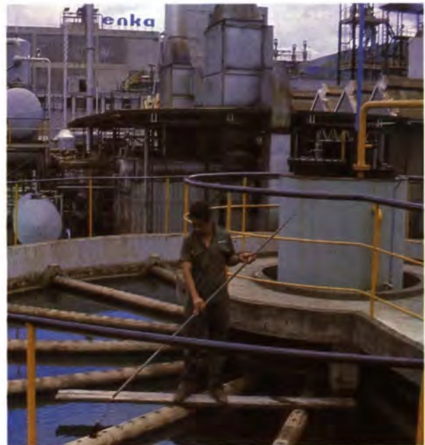
Cleaner performs maintenance work on waste-water purification plant at Enka de Colombia's fiber manufacturing facility at Medellin.
