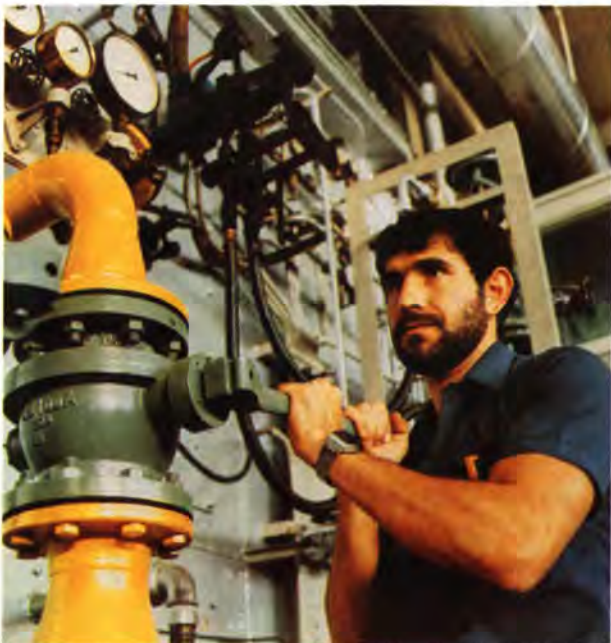
» Technician in power plant of La Seda de Barcelona opens valve in the oil supply line to the boiler house.
